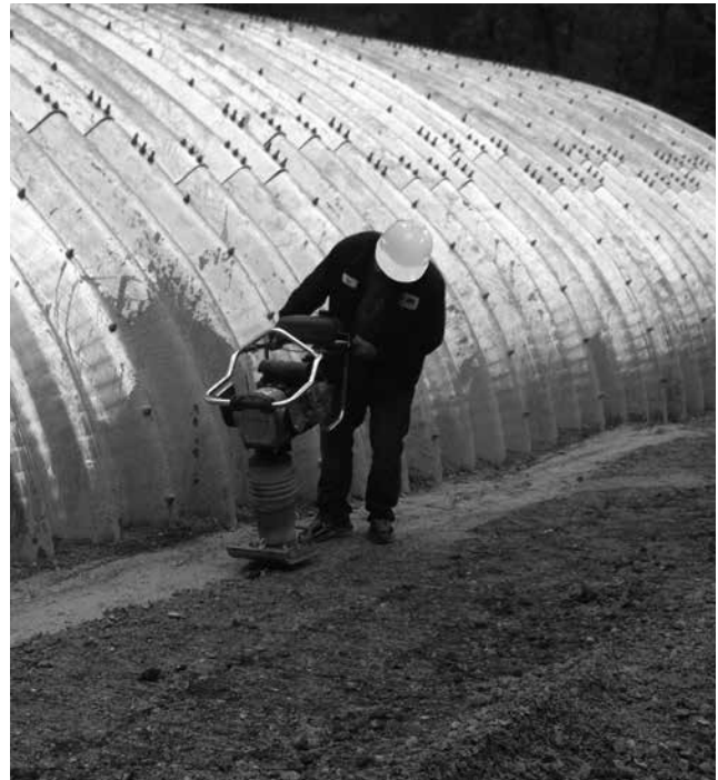
Typically, each lift shall be compacted to a minimum of 90 percent density per AASHTO T 180.
